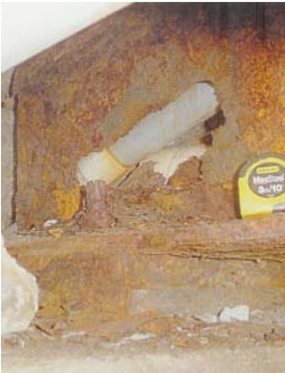
Figure 5: 100% section loss to stringer (Source: DCR 2006 Inspection Report)
