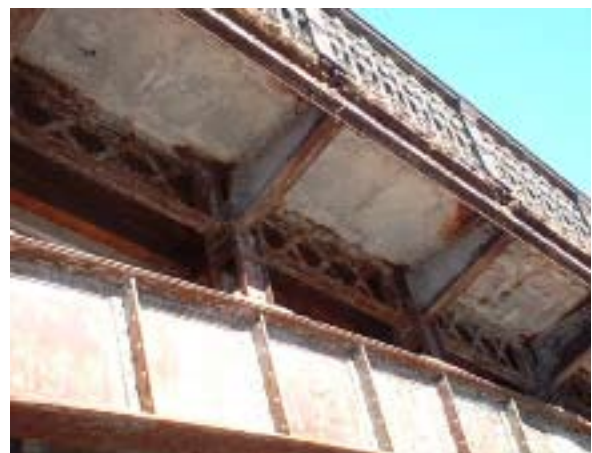
Figure 4: Beams (perpendicular to bridge) and Stringers (sections with “x” bracing) (Source: DCR 2006 Inspection Report)
